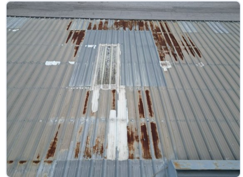
09 Corrosion advancing at the end laps, with silicone applied over a translucent light panel and the panels around it.
