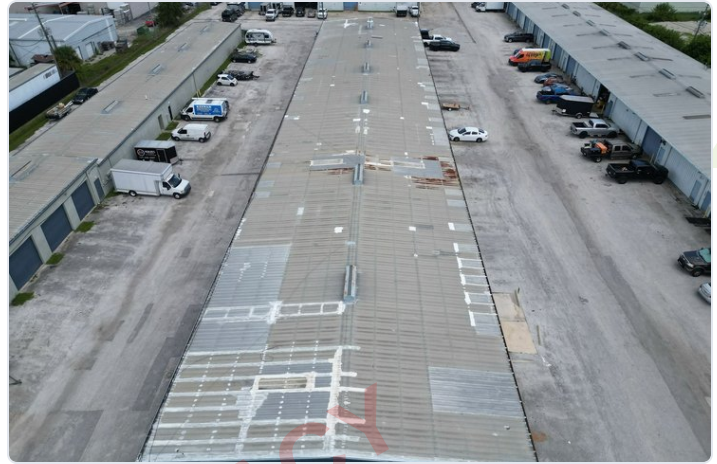
06 Opposing view — the density and spread of the repairs, with rust staining visible at the end-lap lines between them.
