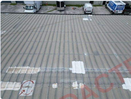
07 Silicone applied along the end-lap lines, with a leak location marked in paint by on-site maintenance.
