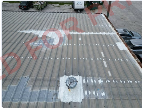
08 Fastener heads individually dabbed with sealant, and a heavily encapsulated ventilator curb.
